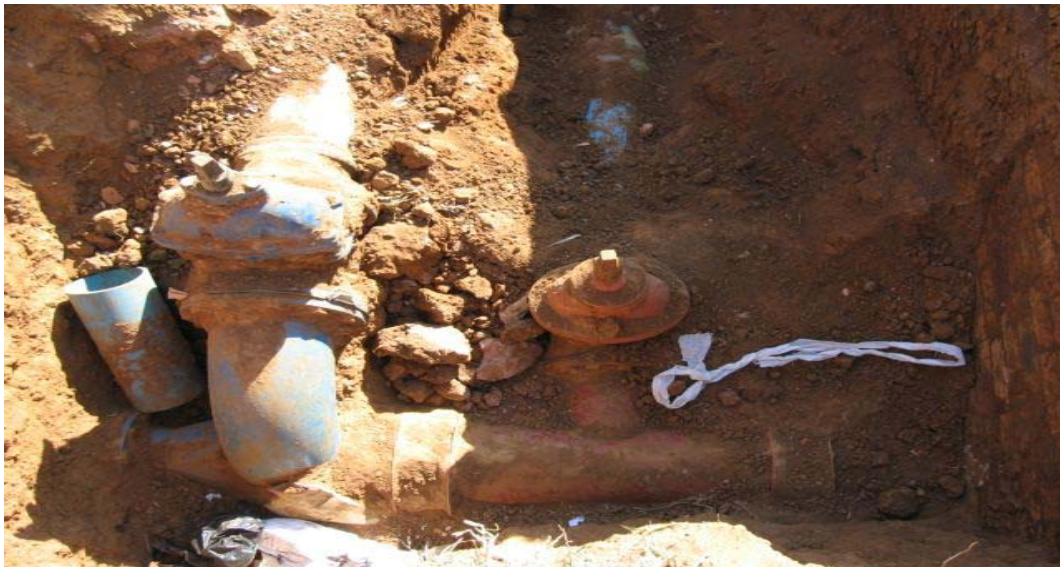
Photo 1.1 – Typical example of an unknown connection
